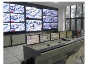
Chongqing University Safe Campus System Project
