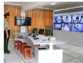
Armed Police Digital Monitoring System
